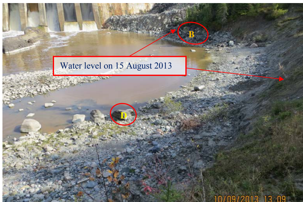
Figure 7: Water level marks and erosion after high flows
