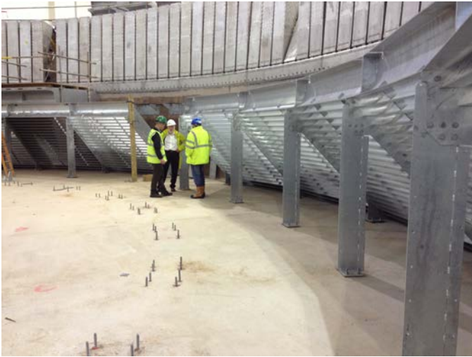
Fig. 8. Installation of the 90° turning vanes, with the wave-makers erected on the step, the bolts in the floor mark the locations of the flow drive units..
