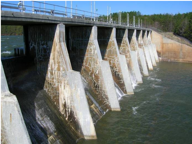
Figure 3 – Pattern Cracking of Piers
