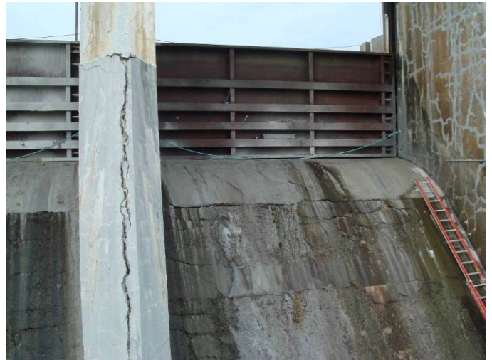
Figure 4 – Cracking of Mass Concrete and Piers
