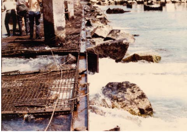
Figure 3. - Damage to the Nimbus hatchery rock weir after a flood event. This is costly and requires emergency action to get it repaired in time for spawning season. (Note: Flow is from left to right.)
