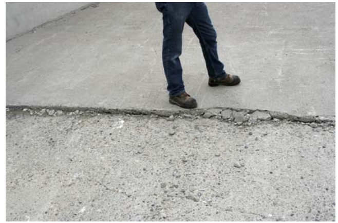
Photo 4: Up thrust on spillway mud slab joint.
