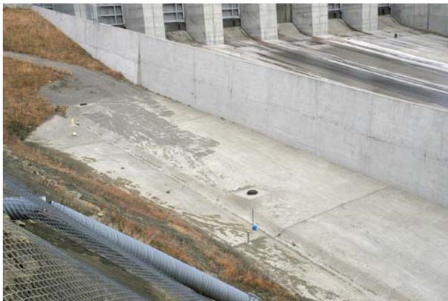
Photo 7: Right side of spillway showing drain manholes, extensometers (yellow; middle left) and SI (blue).
