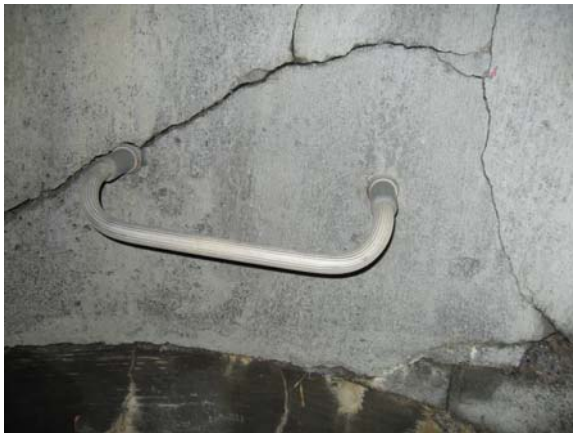
Photo 5: Cracking in drainage manhole barrel.
