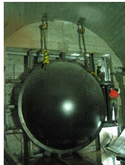
Figure 5: Headrace Access Door
