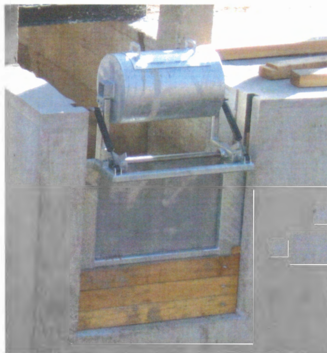
Figure 2. ITRC Flap Gate Installation at Walker River Irrigation District (ITRC, 2012)
