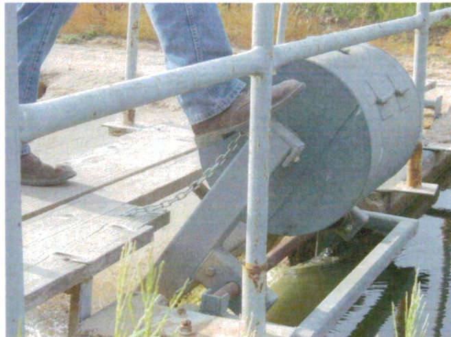
Figure 23. Chowchilla Water District chain stops (ITRC, 2013)
