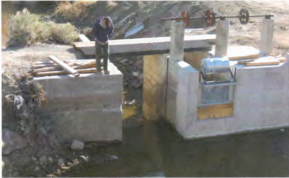
Figure 21. ITRC Flap Gate Installation on WRID Saroni Canal Headworks (ITRC, 2013)
