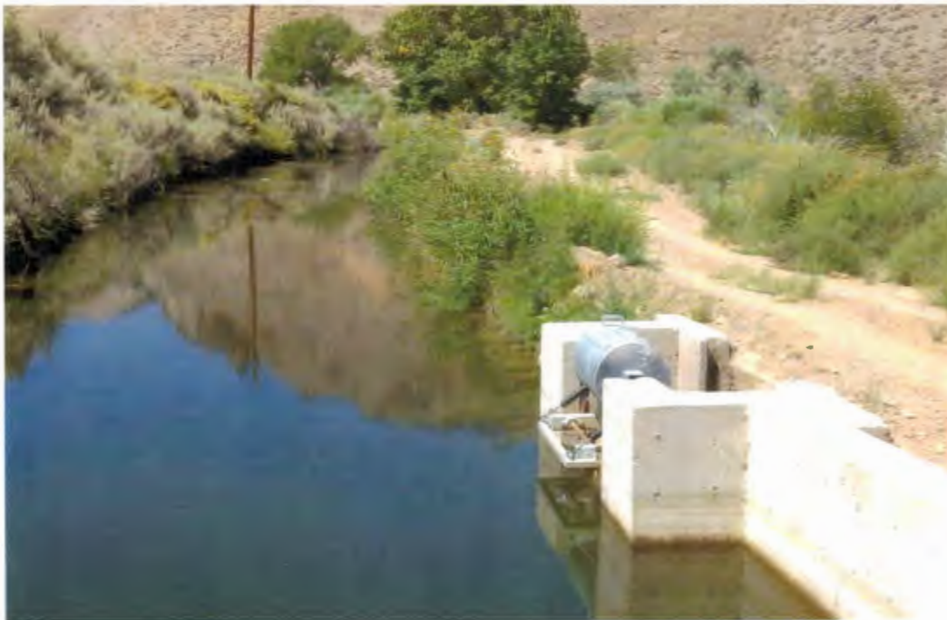
Figure 22. ITRC Flap Gate Installation on WRID Plymouth Canal Headworks (ITRC, 2013)
